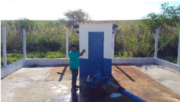
POÇO 2 (VICINAL) – 7449,502 S; 629,873 E
